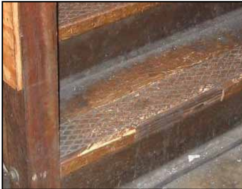
The repair of damaged stairs needs to be a top priority.
