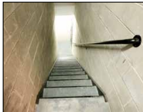
Maintaining adequate lighting is especially important in stairways. This stair needs additional lighting to help staff see each stair clearly.
