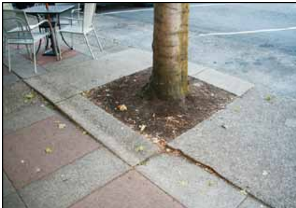
Raised concrete, pavers, and bricks create a trip hazard. Tree roots can raise sidewalks and walkways when a tree is planted too close.
