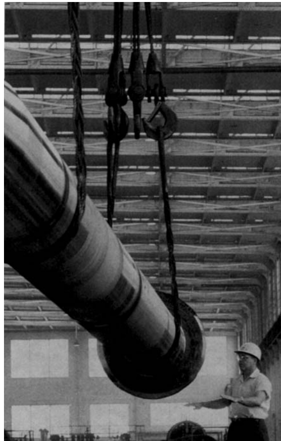
Figure 2. Braided slings are resistant to kinking. Be sure loads are hoisted uniformly and all slings have a minimum safety factor of five.
