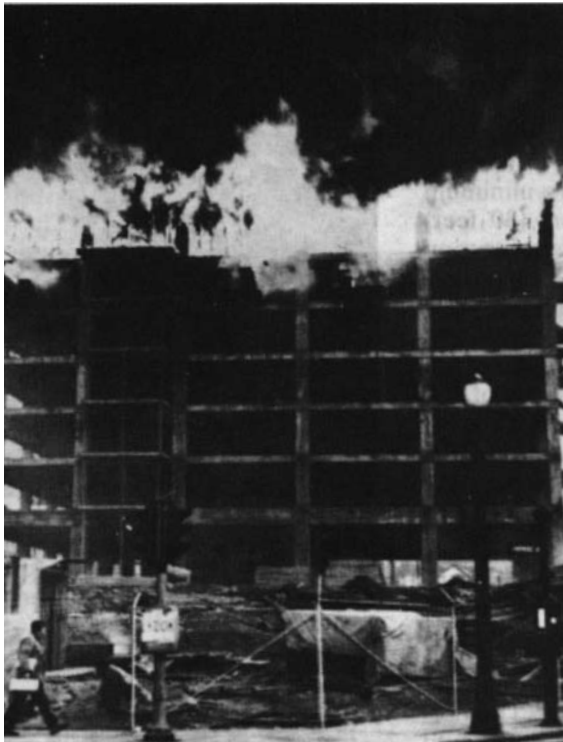
Figure 5. Blaze caused by a faulty heater backfiring and setting the scaffolding and other timbers afire on this partially constructed apartment building. Note: Fire alarm is attached to lamppost.
