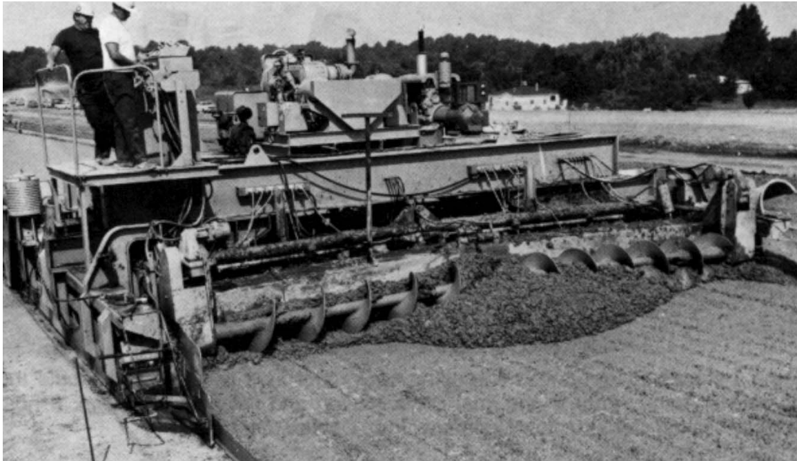
Figure 2 shows a slip-form paver as it consolidates, screens and finishes the concrete.
