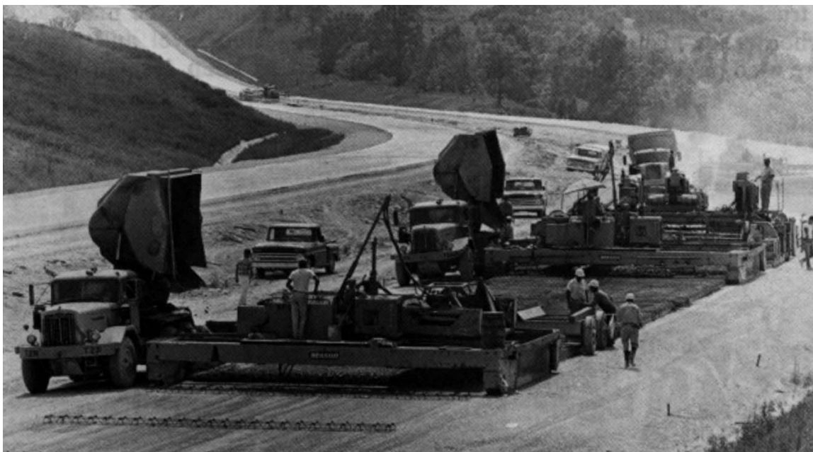
Figure 1 shows self-propelled spreading equipment as it is used to distribute the concrete uniformly prior to the final consolidation and finishing operation.
