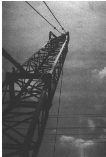
Figure 3. Crane with hoist cable 13½ ft from power line as viewed by crane operator.
