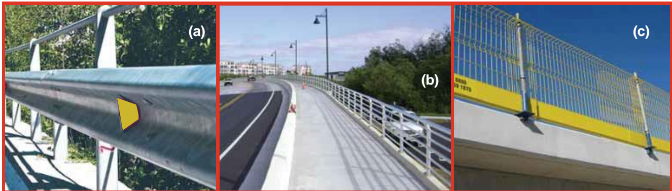
(a) Existing bridge guardrails may not meet OSHA requirements. This guardrail is too short and lacks toeboards. Photo source: NBC. (b) This existing guardrail appears to meet OSHA requirements. Photo source: BravoFence. (c) When existing guardrails are not adequate or are not in place, then temporary guardrail can be installed. Photo source: J-Safe.
