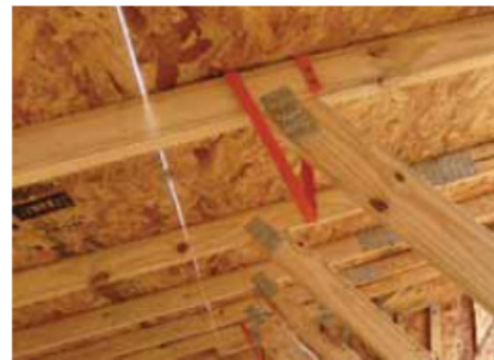
A pre-installed attic anchorage system.
