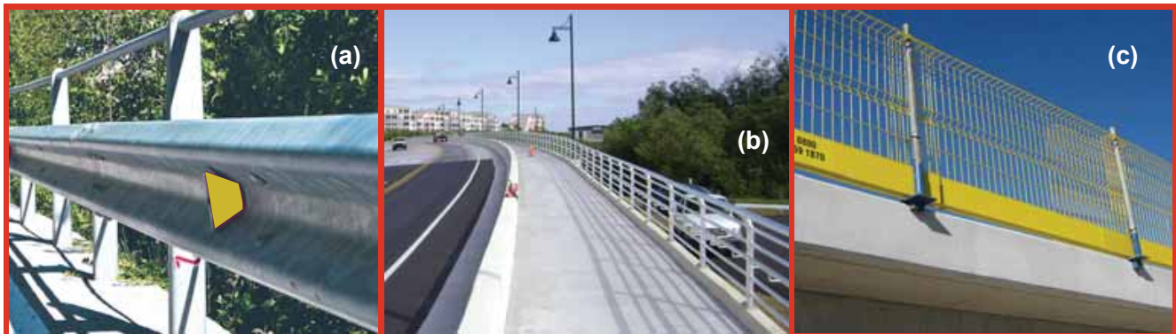
(a) Existing bridge guardrails may not meet OSHA requirements. This guardrail is too short and lacks toeboards. Photo source: NBC. (b) This existing guardrail appears to meet OSHA requirements. Photo source: BravoFence. (c) When existing guardrails are not adequate or are not in place, then temporary guardrail can be installed. Photo source: J-Safe.
